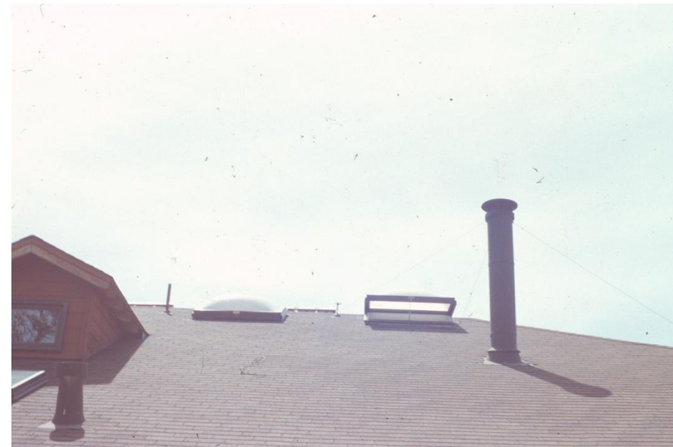
Operable skylight open on upper roof to induce air flow and passive cooling in summer
