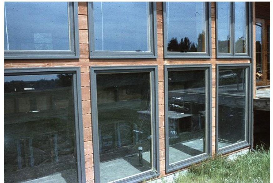
Glazing of crawl space under living room for water filled 19 Liter black metal cans for thermal storage
